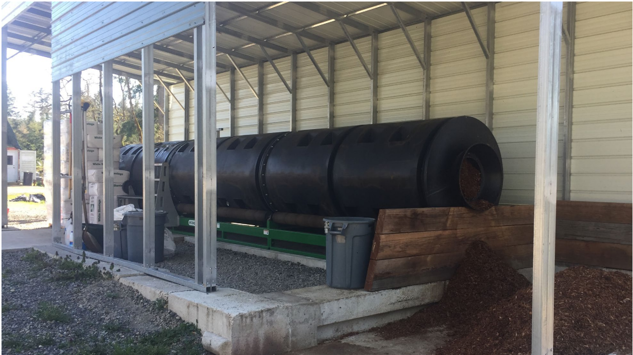
Figure 12. In-Vessel Ecodrum™ Composter with forced air system. Source: Ecodrum™ Composters.
